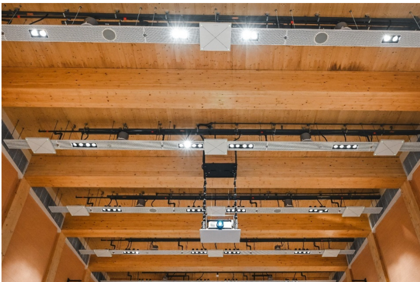
10 units of TCC 2 were installed in the ceiling across the theatre-style seating area for audience pickup.
